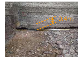
▲⑦洗掘(深さH=0.4m)
